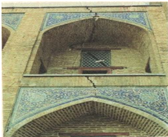
Picture 2. Through crack on second floor western part (western part of facade – first khujra)
